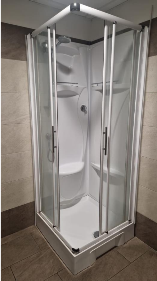
Figure 7 one of the showers at the via Sommarive 18 site
